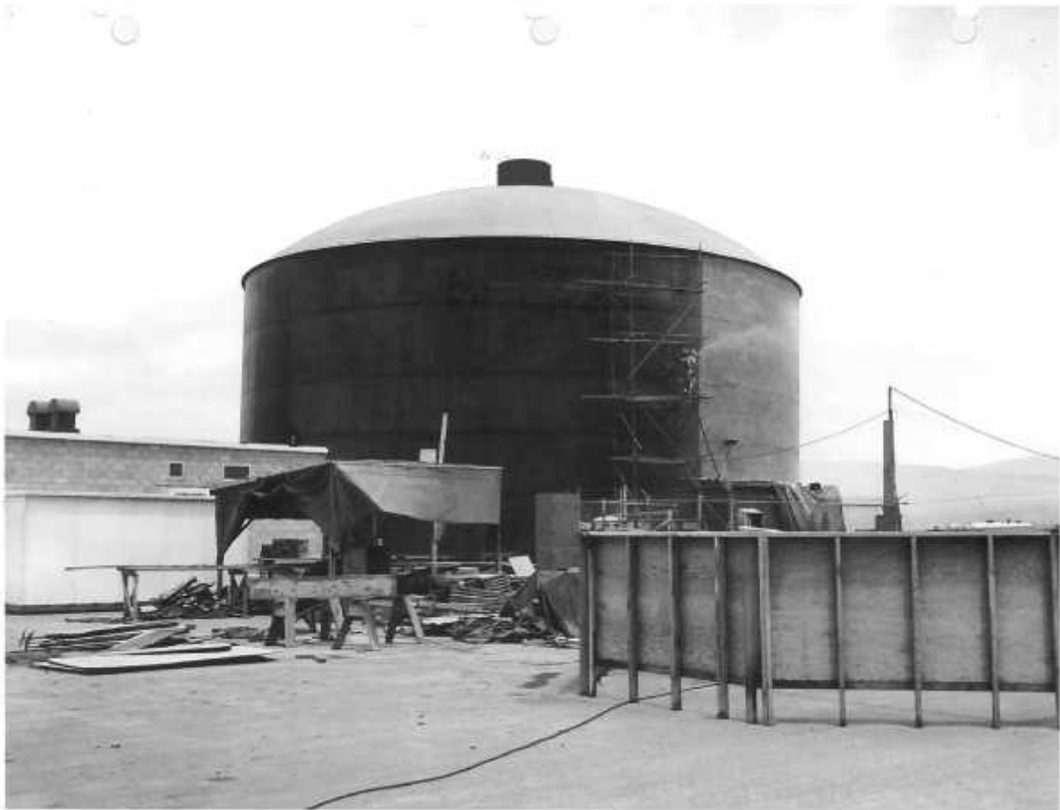
Figure 5. Building 280 construction nearing completion. Note scaffolding and worker spraying on mastic material finish at the exterior, 1956. LLNL Archives.
