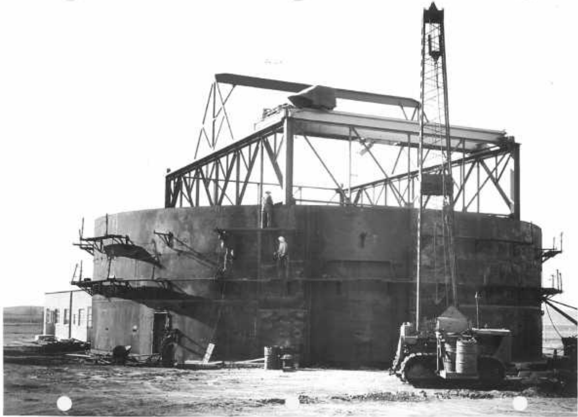
Figure 4. Construction of the steel plate wall structure around the 15-ton traveling crane, 1956. LLNL Archives.
