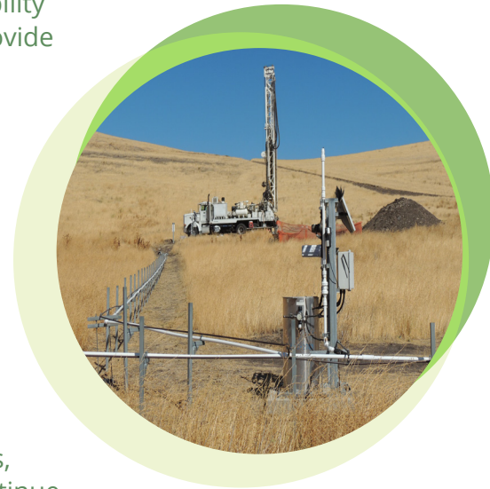
Wells at Site 300 are used to monitor groundwater quality
