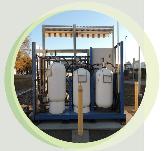
Livermore Site treatment facility
